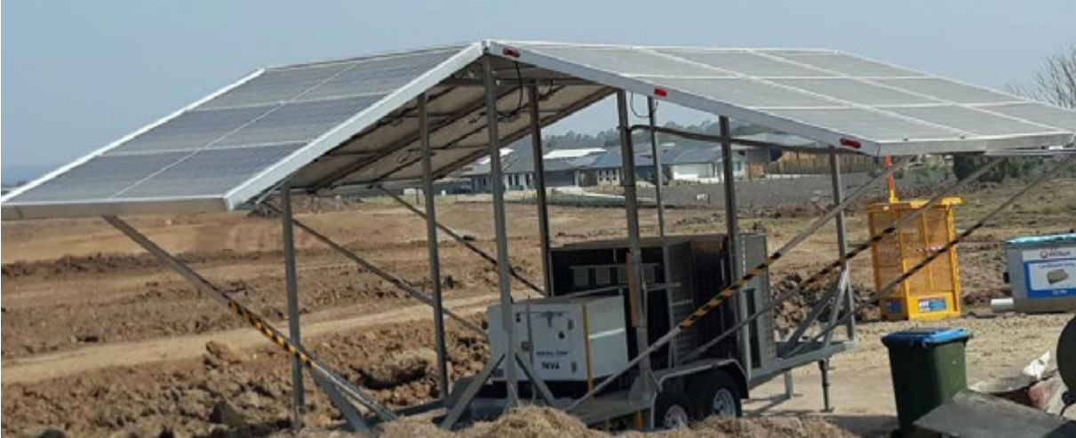
The solar panel initiative on a BMD Urban project in South East Queensland
